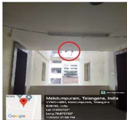
Camera Installed In the Corridors
