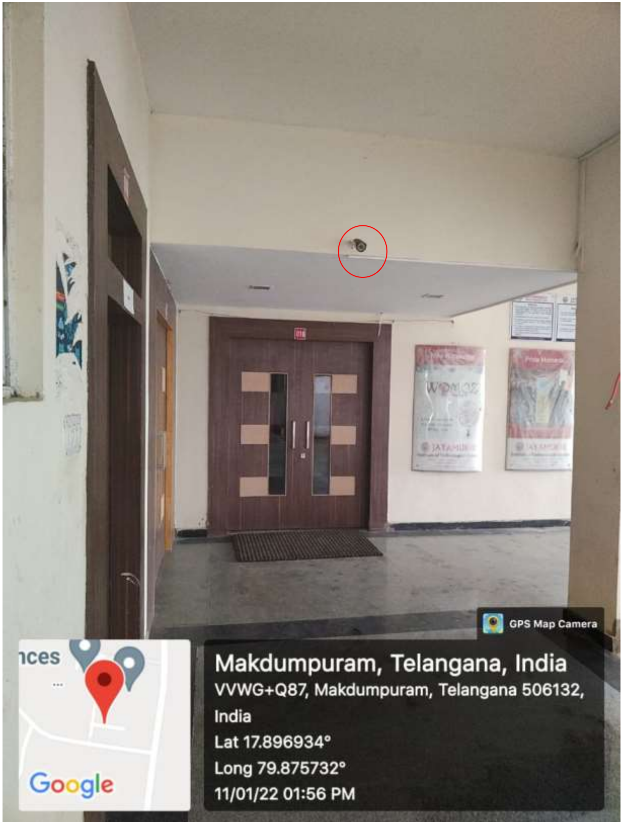
Camera Installed In the Auditorium
