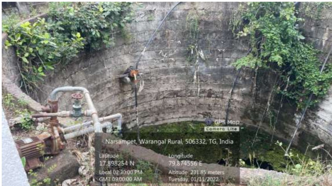
Open wells connected with motor to supply water to different areas.
